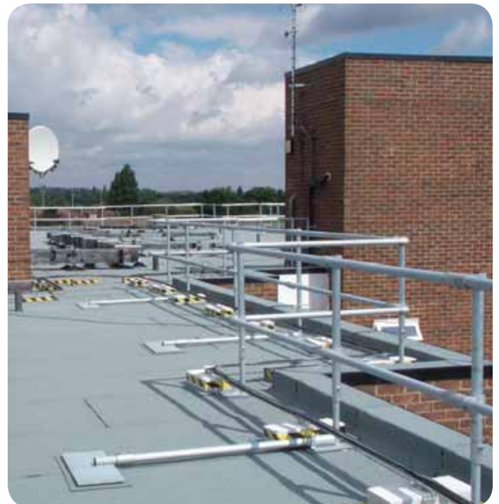
▲ Edge protection provided by free-standing handrail system
