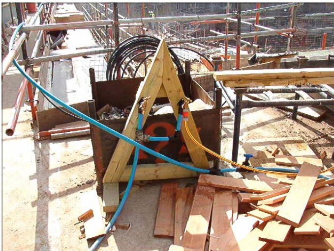
An example of a temporary watering system rigged up on site to provide an adequate mains watering feed to different roof areas.
